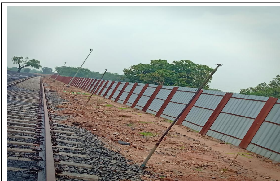
Water sprinkling system at Gajra Bahra Coal siding
